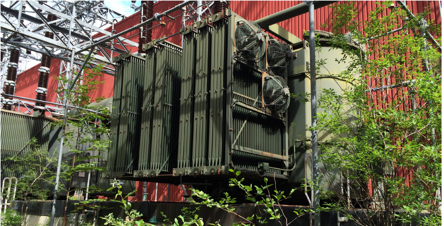
A transformer at the Twin Falls plant which has been removed and sent for disposal at an approved PCB disposal facility.
