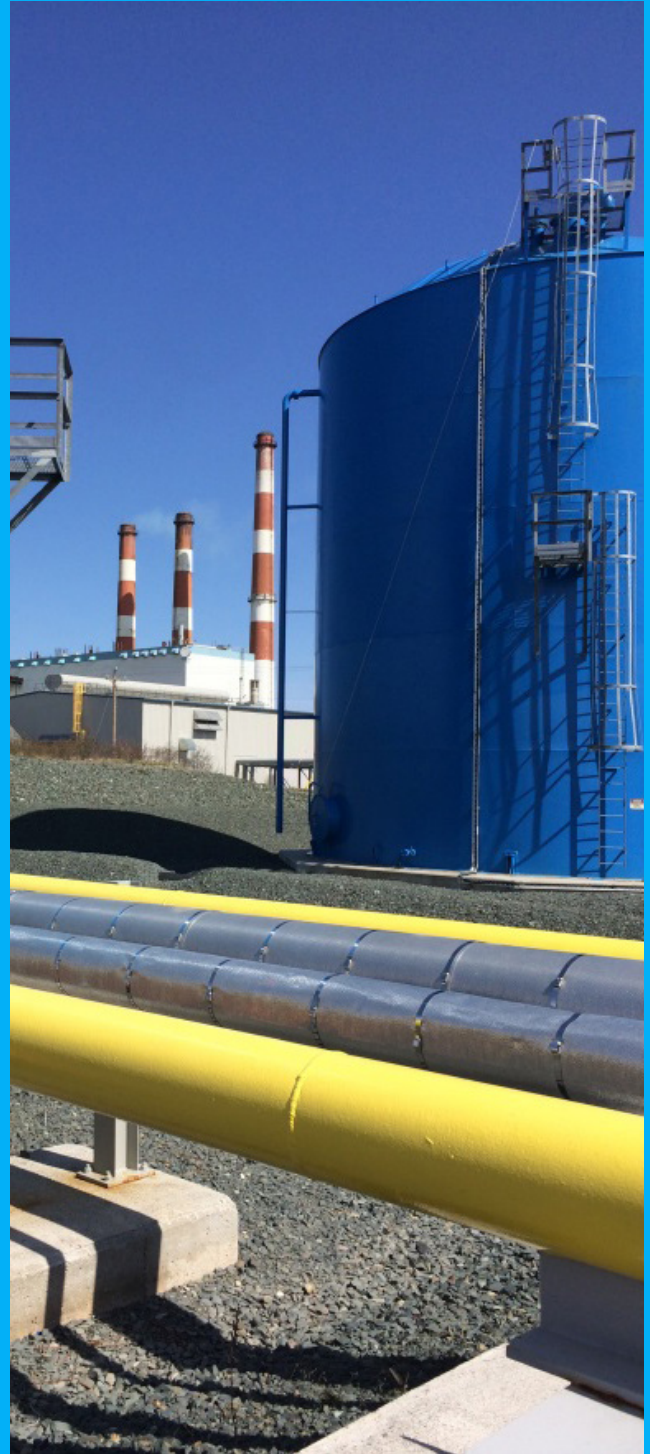
The Holyrood Thermal Generating Station generates between 15 to 25 per cent of the island's electricity each year.
