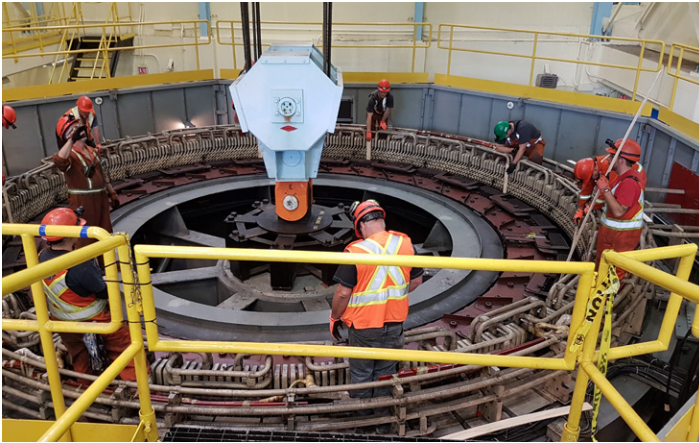
The largest generating unit at Bay d'Espoir undergoes preventative maintenance to ensure long-term reliability.
