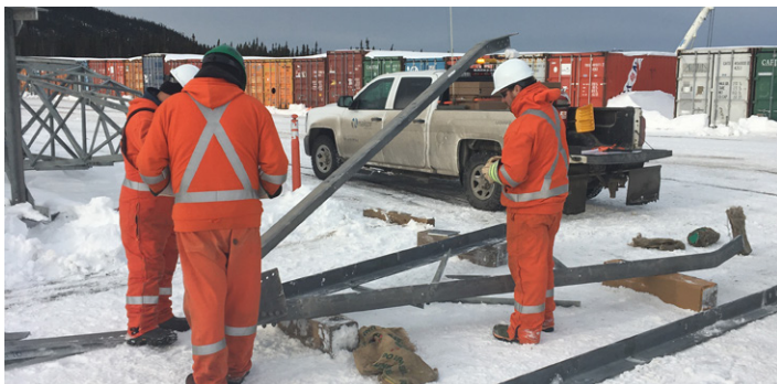
The LIL stretches across many remote areas of Newfoundland and Labrador. Emergency planning exercises are critical to ensure the safe operation of our assets.
