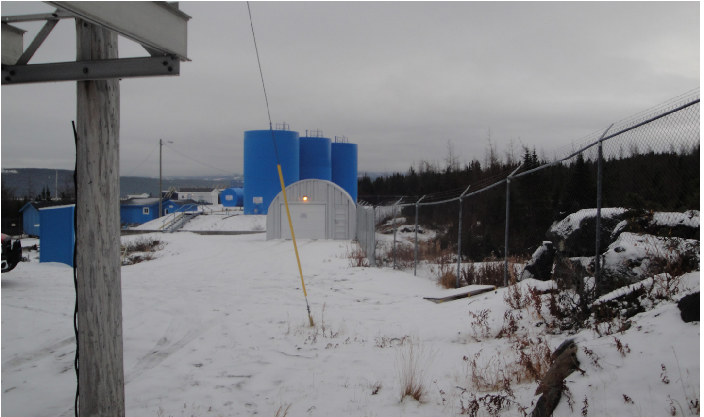
The Makkovik Diesel Plant.
