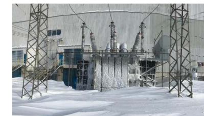
Due to the extreme volume of snow that fell during the blizzard, electrical equipment at many sites, like the transformer shown above in Holyrood, quickly became covered in snow.
