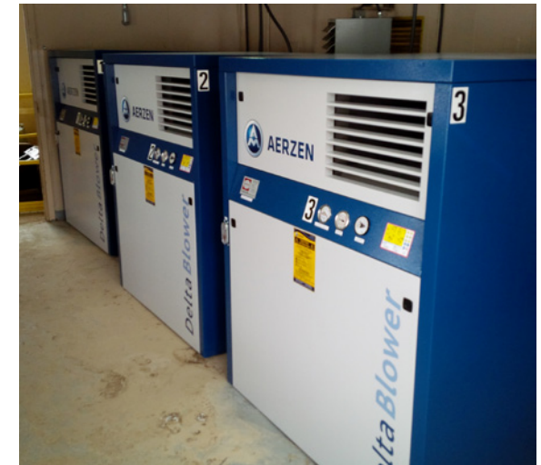
Aeration Tank Blowers.
