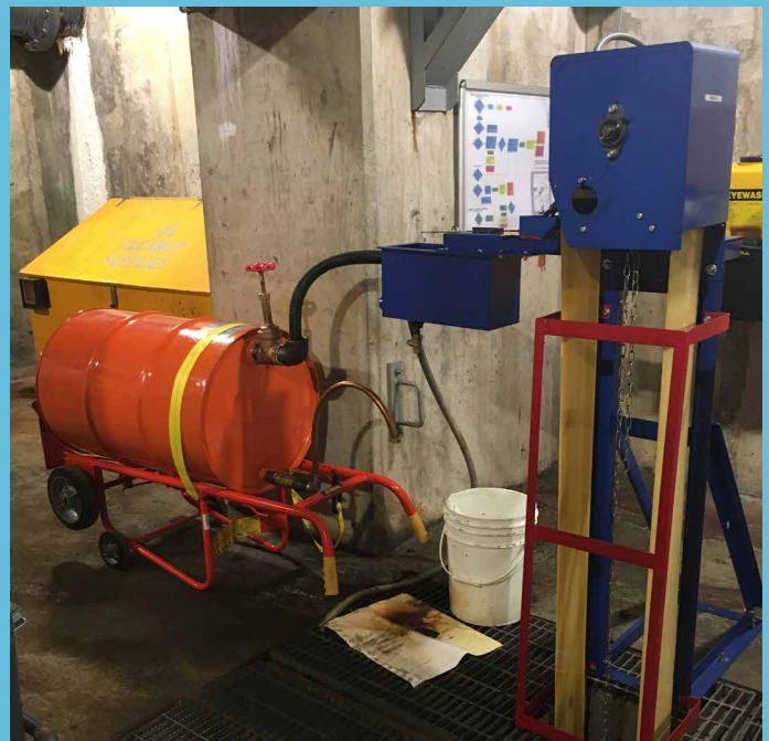
Churchill Falls drainage gallery sump oil-water separator system.
