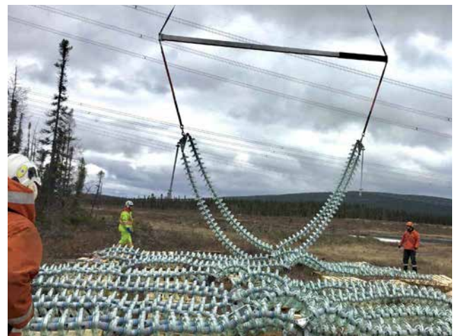
Since 2018, old ceramic insulators (top) have been removed from our 735 kV transmission line and replaced with new strings of glass insulators (bottom).
