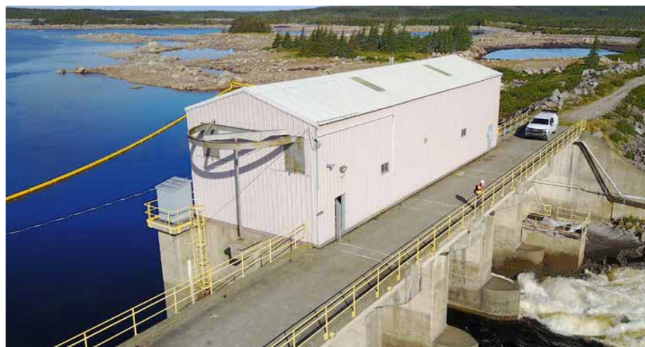
Work began in 2021 on refurbishment of the Ebbegunbaeg control structure, part of the Bay d'Espoir hydroelectric system.
