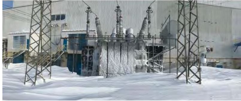
Due to the extreme volume of snow that fell during the blizzard, electrical equipment at many sites—like the transformer shown above in Holyrood—quickly became covered in snow.
