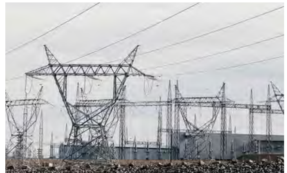
TOP: Muskrat Falls powerhouse. BOTTOM: Transmission towers and electrical yard at the Muskrat Falls site.
