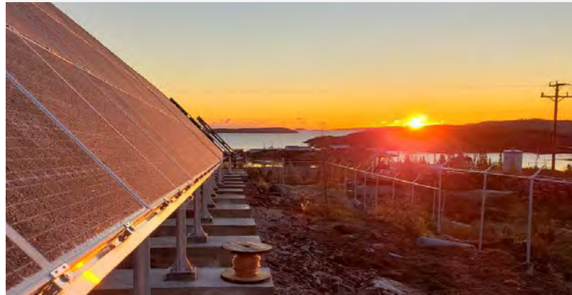
The sun rises over the St. Mary's River Energy solar farm, ready to produce and store energy for use in the community.
