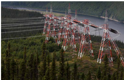
The 735 kilovolt transmission lines span 1,829 m (6,000 feet) over the Churchill River
