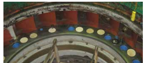
Top: The bushings at Bay d’Espoir machined and ready for installation.
