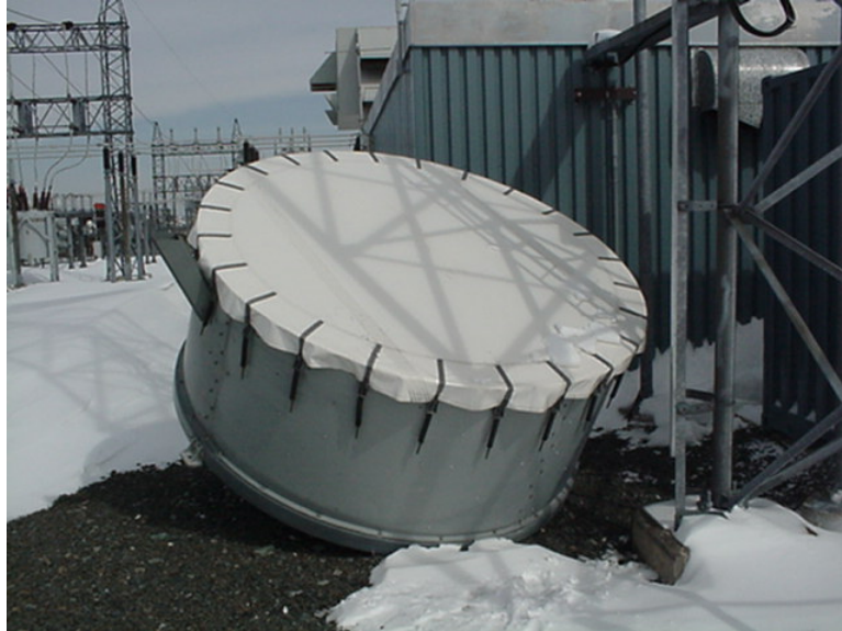
Figure 1: Microwave Antenna with Radome
