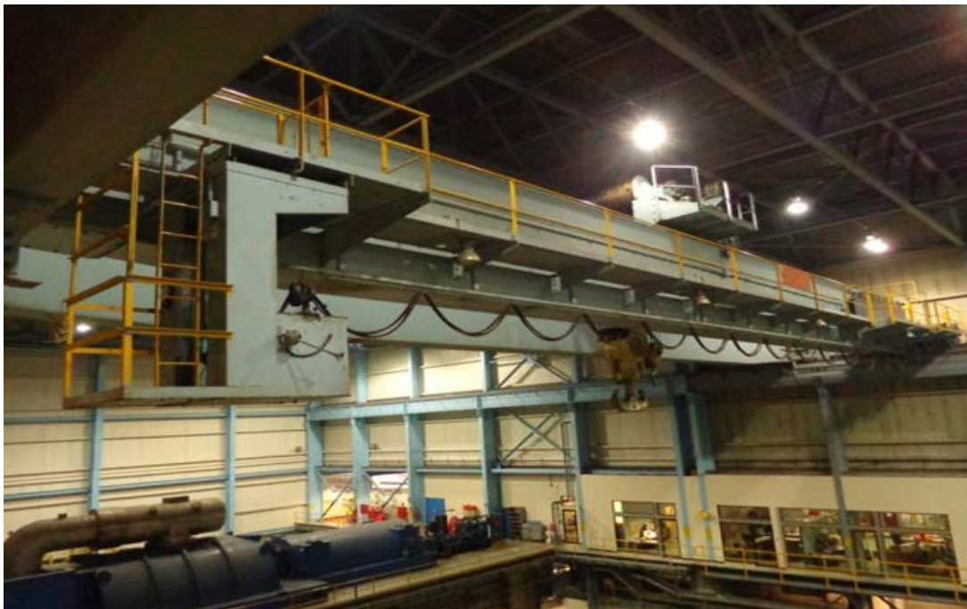
Figure 1: Overhead Crane 1 in Holyrood Powerhouse Turbine Hall
