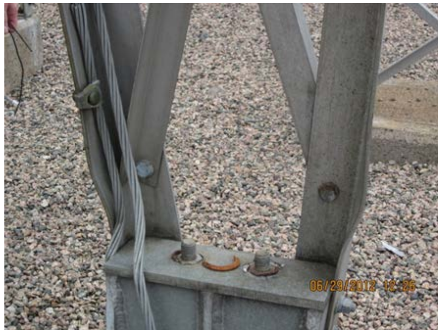
Figure 3: Example of Deformation of Aluminum Structure Legs as Result of Uplift Stresses
