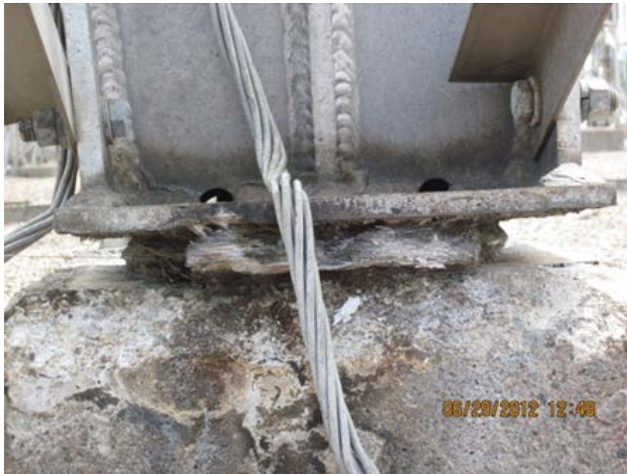
Figure 1: Example of Aluminum Oxide Formation between Concrete Surface and Aluminum Baseplate
