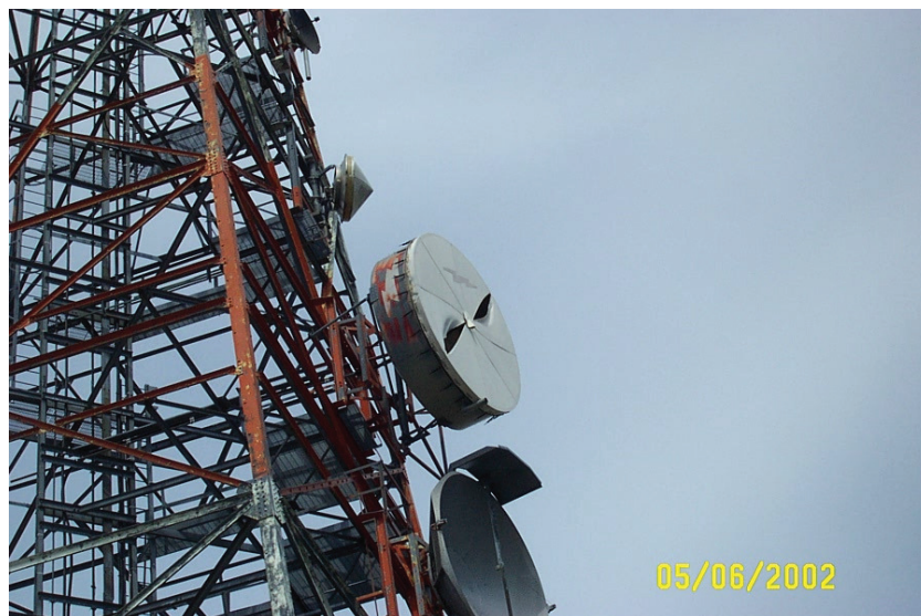
Figure 3: Heavily Damaged Radome
